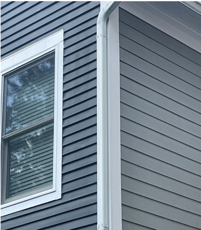
Figure 11. The thickness of the wood siding on the front (left) creates a deeper shadow line than is achieved with the fiber cement siding used on the side (right) elevation. While the exposure can be adjusted, fiber cement siding is not available in a matching thickness. Photo: John Sandor, NPS.
